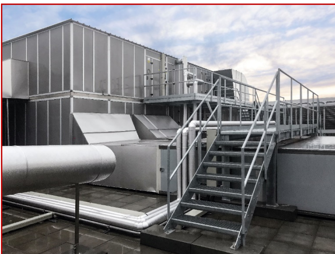
Large rooftop installation – a high-performance WEGER ventilation system ensures ideal conditions for shoppers at the Mall of Switzerland.
